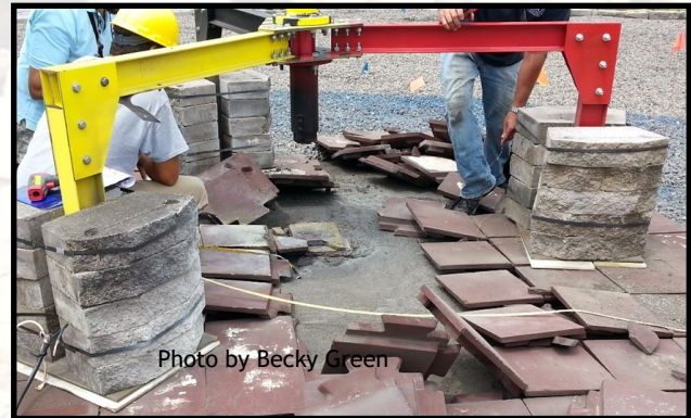
The pad after the motor burn
